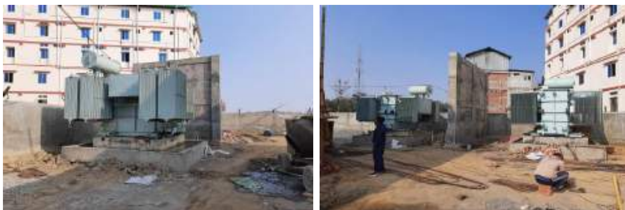
Fire Wall at 33/11 kV new sub-station at Pishum (GIS)
