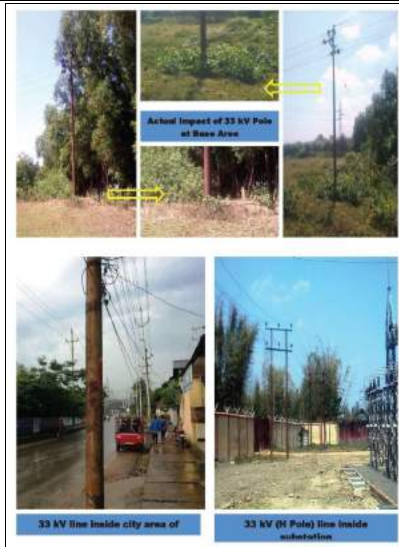
Figure 5.2: 33 kV Lines (Single & H Pole) Depicting Base Area Impact
