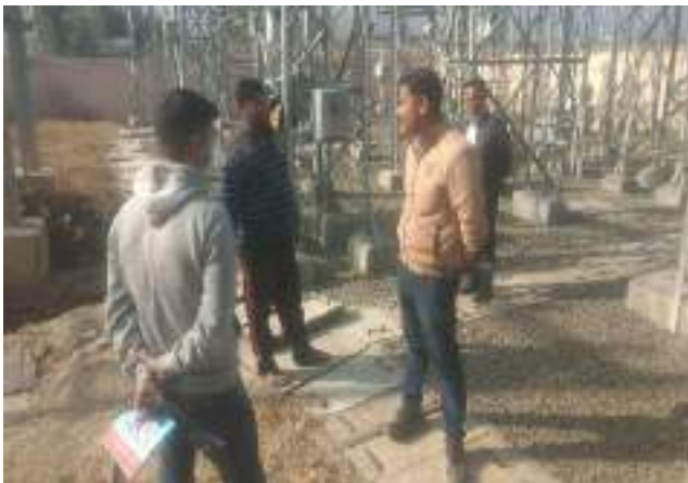
33/11 kV Kwakta Sub-station
