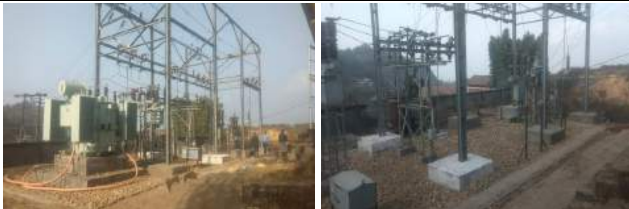
Existing 32/11 kV Substation at Tamenglong (Augmentation)
