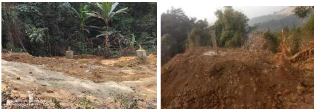
Tower Foundation work at Rengpang and Tamenglong (excavated material has been backfilled)
