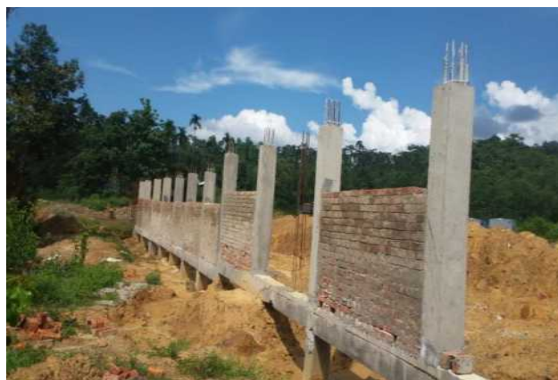
132/33 kV Longnak S/S Boundary Wall
