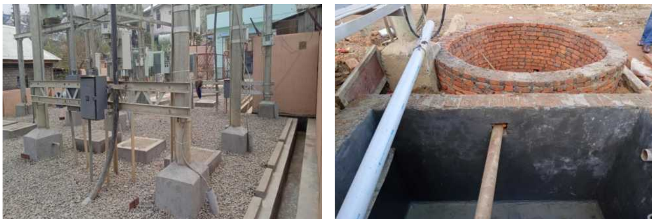
Drainage and Sewage system within the Lalmati (Zubza) Substation
