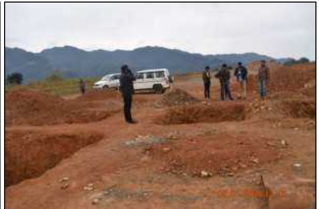
132/33 kV Substation at Zunheboto
