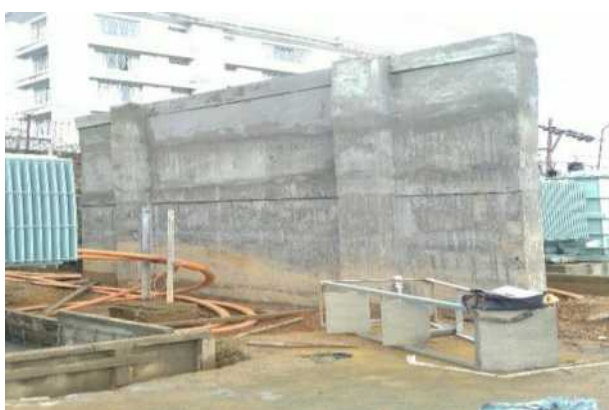
Fire Wall at ITI, Kohima
