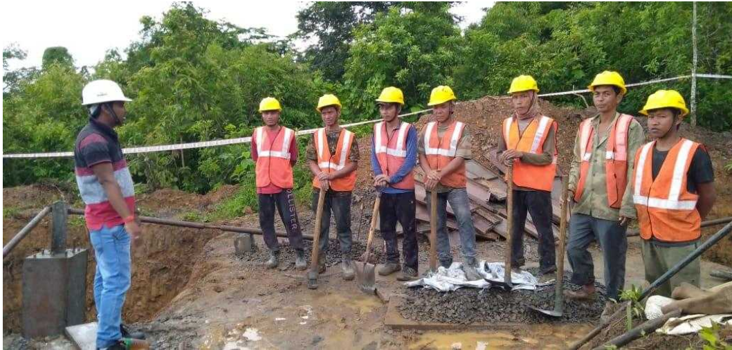
220 kV S/C on D/C Tower New Kohima – Mokochung T/L
