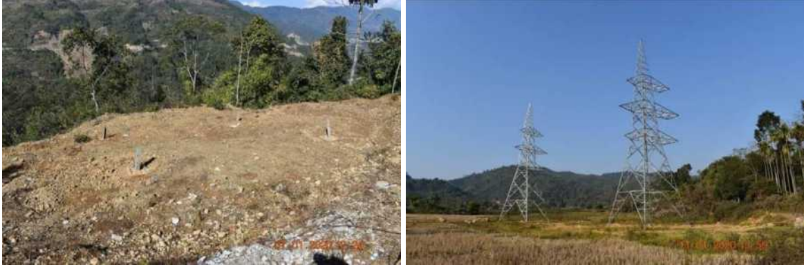
Refilling and leveling of excavated material after tower foundation and erection work
