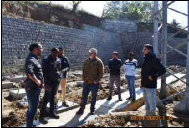
132/33 kV Substation at Wokha
