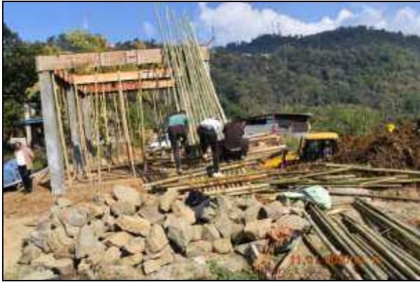
33/11 kV Substation at Mokokchung Hospital Area
