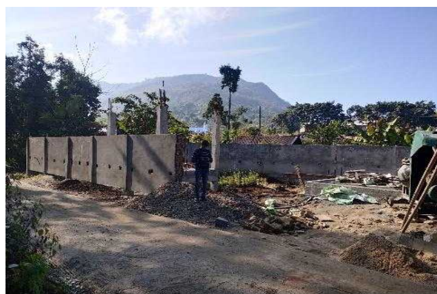
33/11 kV Chukitong S/S Boundary Wall
