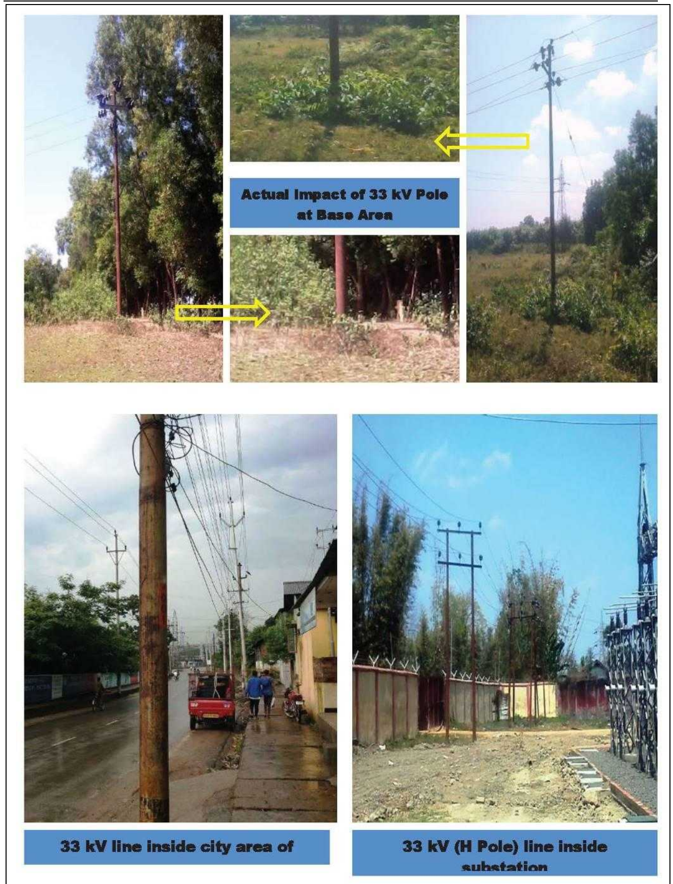
Figure 4.29: 33 kV Lines (Single & H Pole) Depicting Base Area Impact
