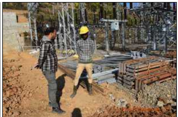
132/33 kV Substation at Mokokchung (State)
