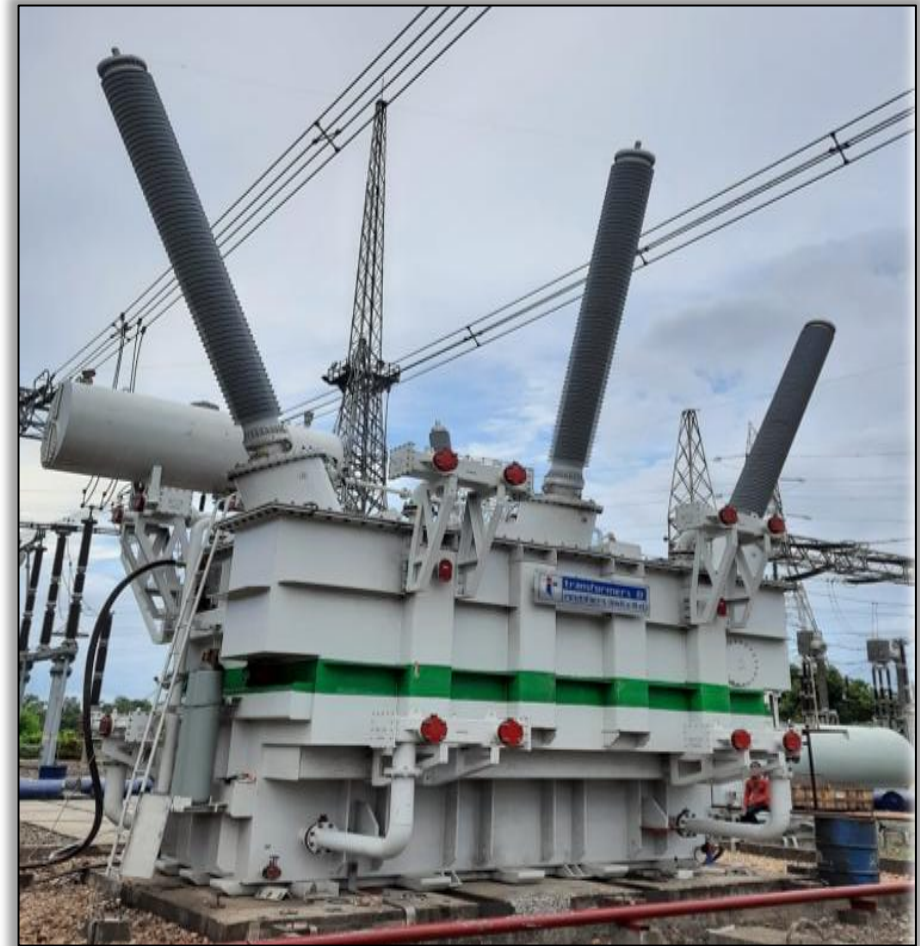
315 MVA, 400/220 kV at HVDC Bhiwadi substation
