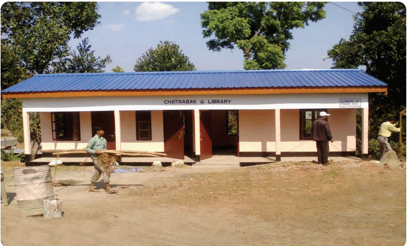
Construction of Chatrabash (Hostel) and Library room at Ramakrishna Mission Hailong, Dima Hasao, Assam
