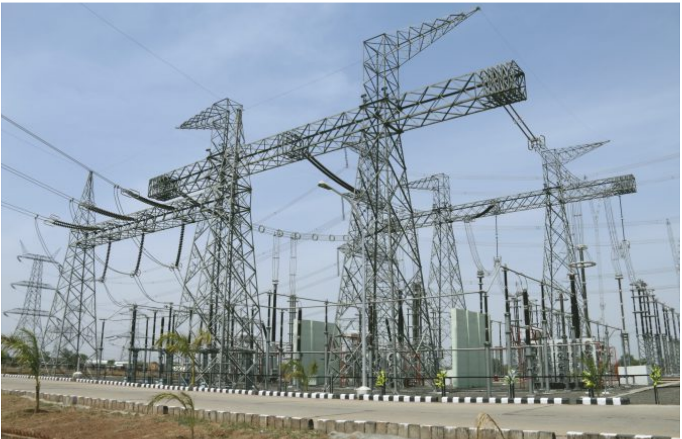
1200 kV Transmission System
