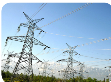
OPGW – Optical Fibre Ground Wire over high voltage transmission line
