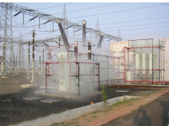
Oil slumps to prevent contamination of ground water
