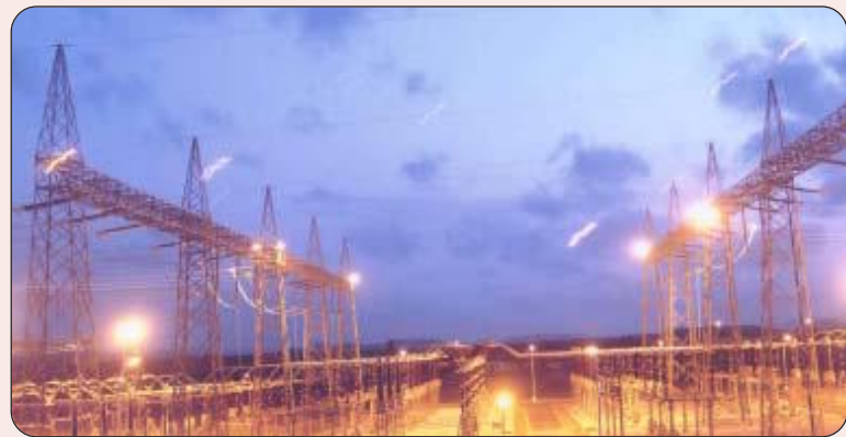
A night view of POWERGRID Substation.
