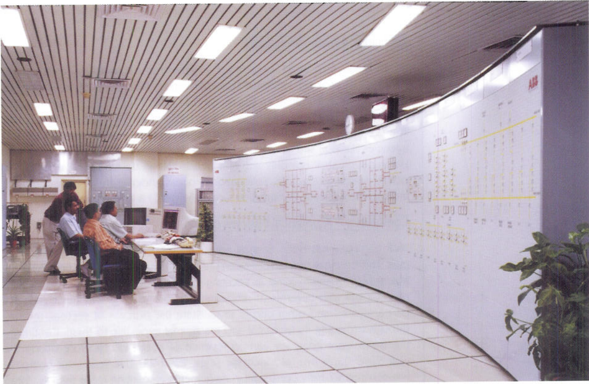
A view of a Control Room
