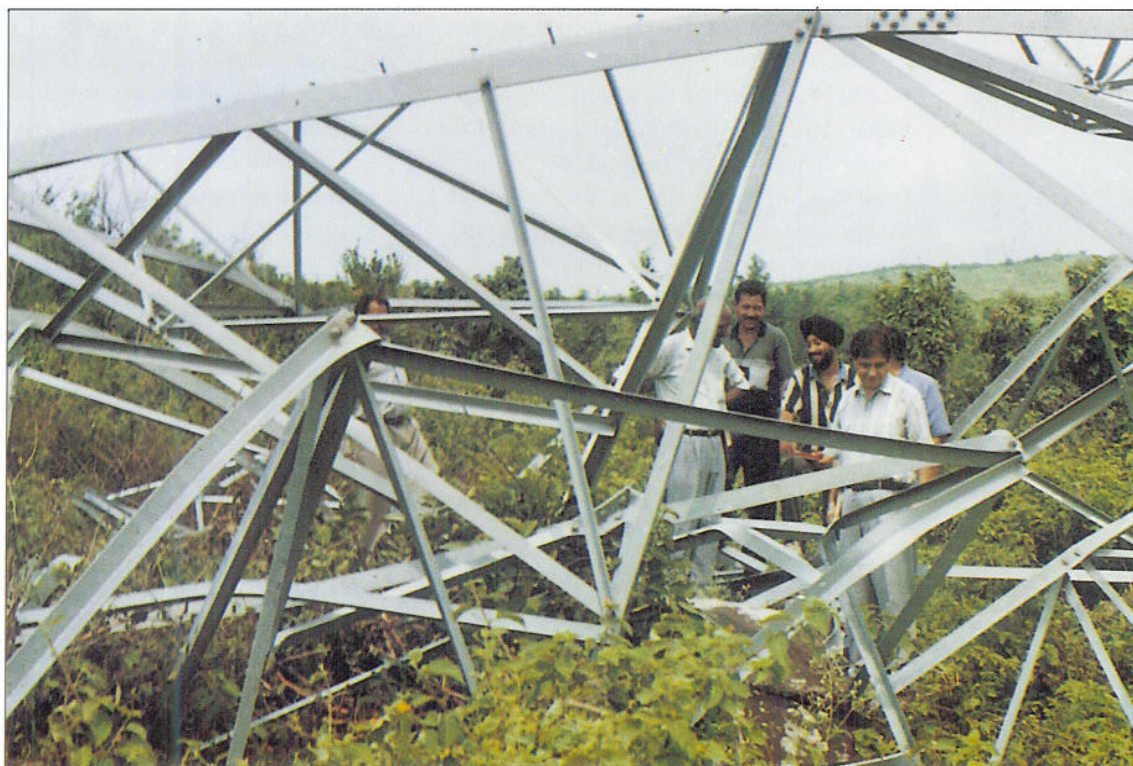
Officers inspecting a blasted tower in Kashmir Valley
