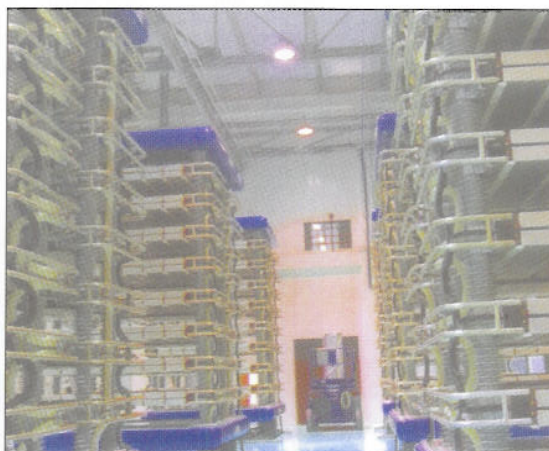
Inside view of Valve Hall in 500 MW Sasaram HVDC B/B station
