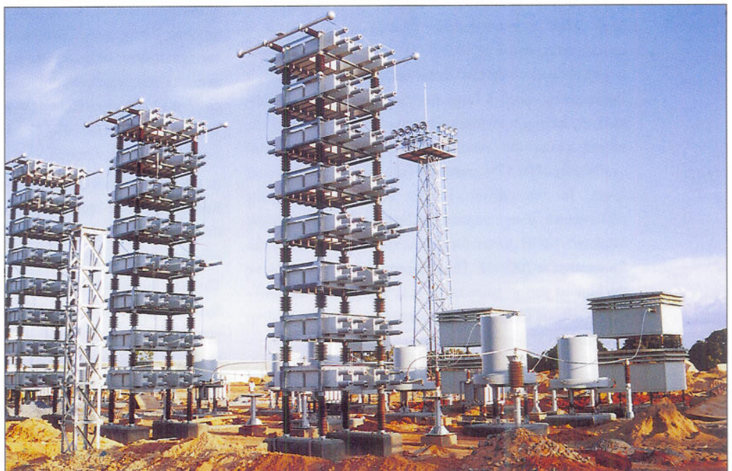
AC filter & Capacitor Bank in Kolar HVDC station
