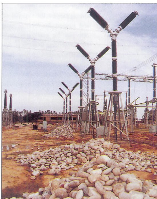
Inter-Pole cable termination & piping of 420 kV CBs
