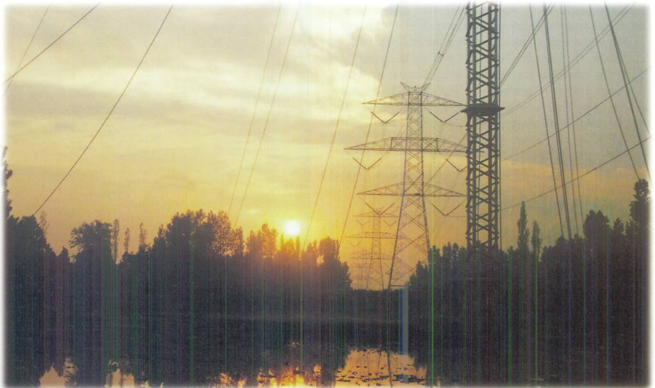
Sunset view of 400 kV D/C Uri-Wagoora line with ERS
