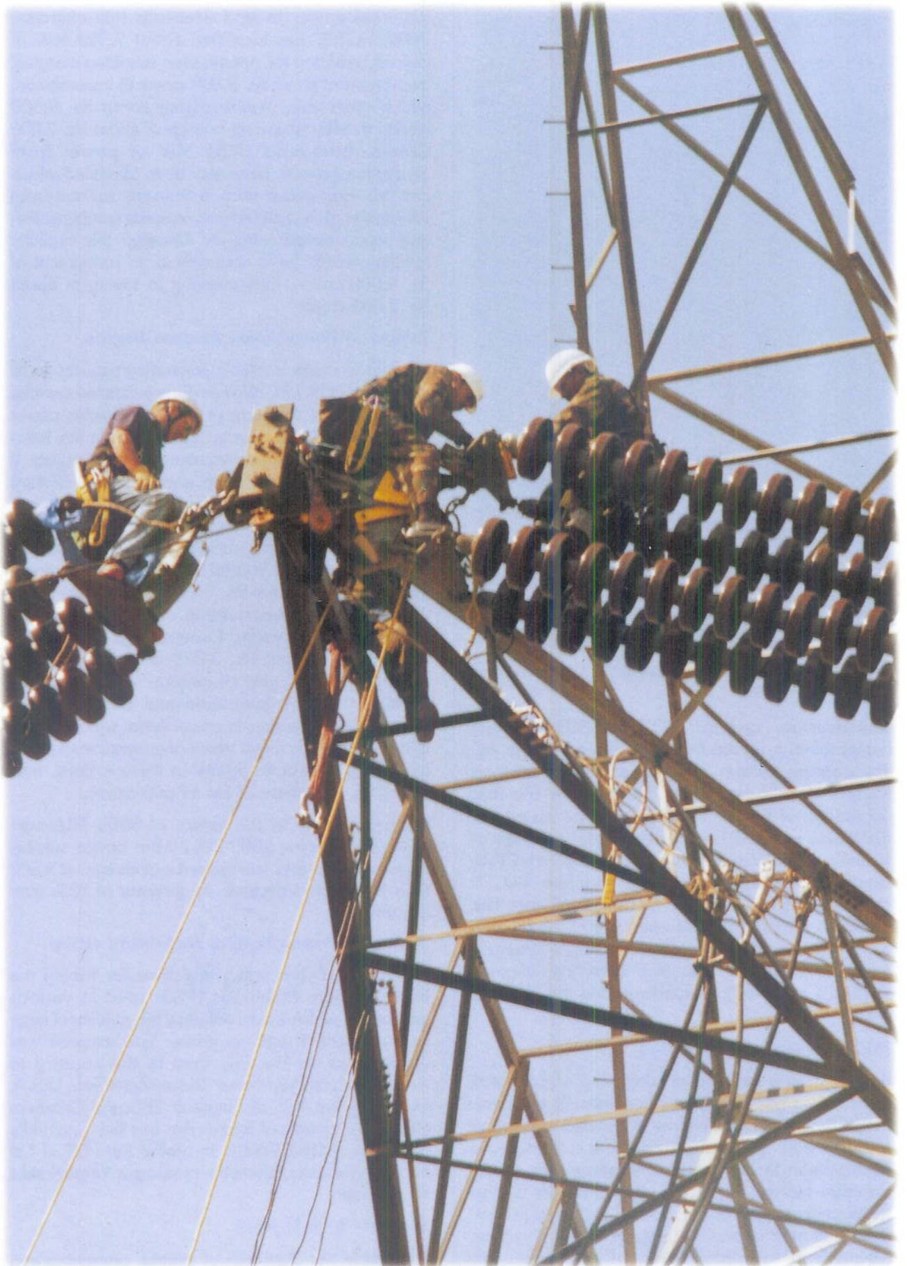
Demonstration of Tension Insulator replacement on HVDC line at Kanpur by NGC, UK
