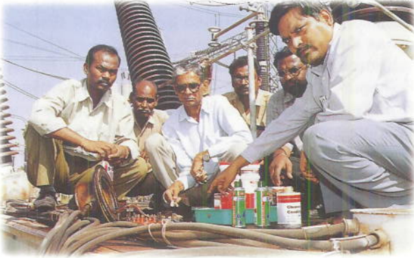
A team from Durg (Raipur) attending the arrest of Oil leakage near CT terminal block in 80 MVAR Bus Reactors of Bhilai-Bhadravati line at Bhilai sub-station
