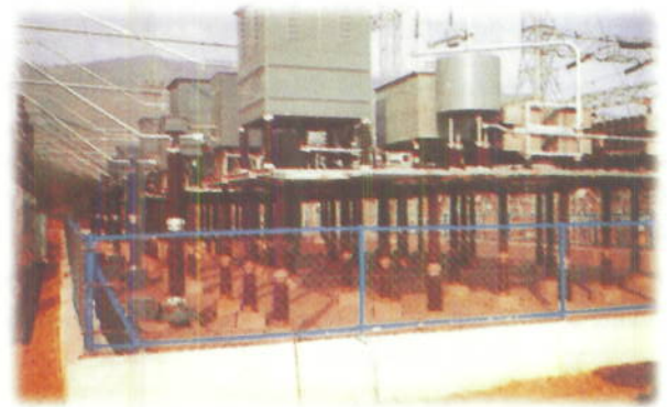
Series capacitors at Kishenpur Sub-station on 220 kV D/C Kishenpur-Pampore line
