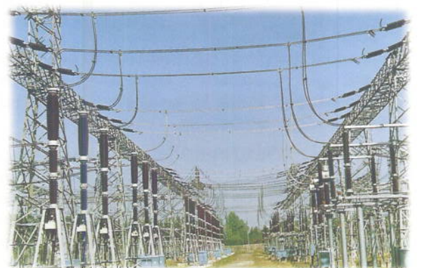
220 kV Switchyard at Wagoora Sub-station
