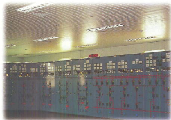
Inside view of Control Room, 400/220 kV Nalagarh Sub-station
