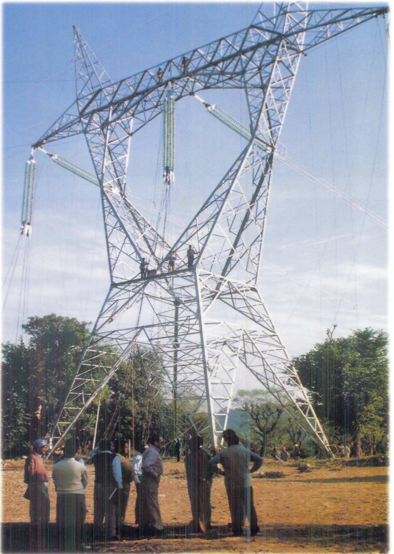
Progress of 800 kV Kishenpur-Moga Line (near Kishenpur) reviewed by World Bank Team
