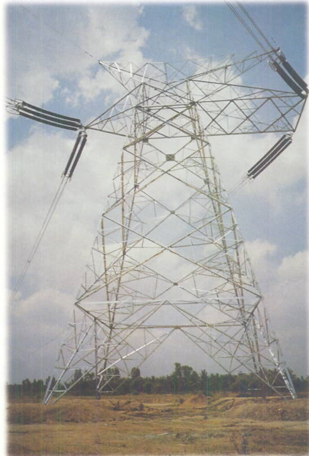
View of erected tower \pm 500 kV HVDC Line in Talcher Transmission System
