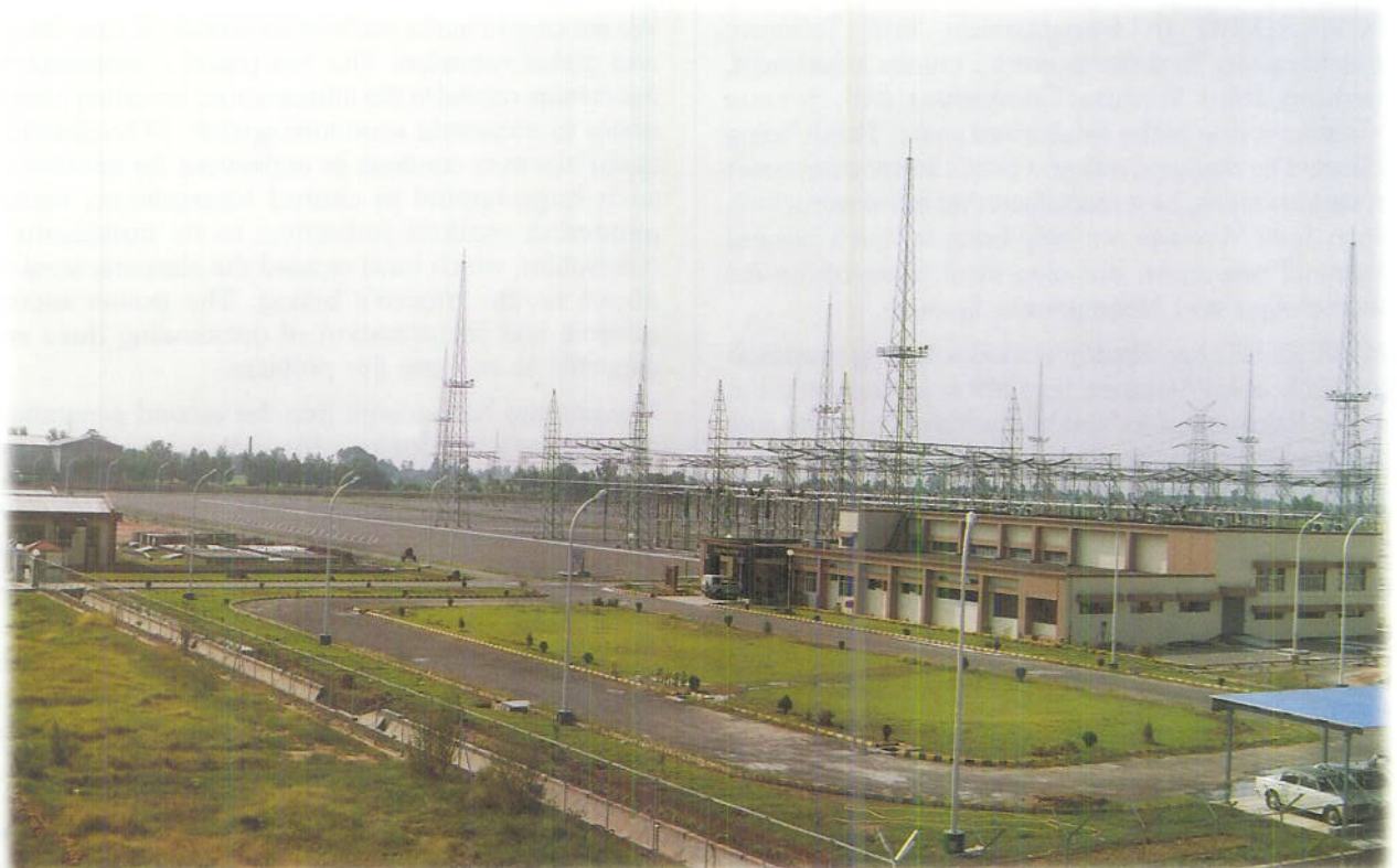
A glance of the new sub-station at Jalandhar
