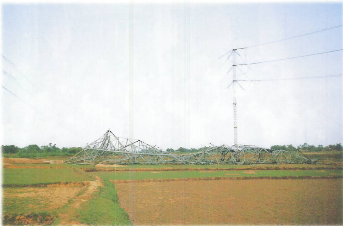
ERS towers with collapsed tower in the foreground while one 400 kV tower is seen in the backdrop
