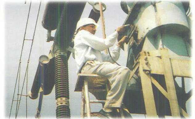
Maintenance team of Bhadrawati Sub-station taking the Tan delta, capacitance measurement of 400 kV CT during AMP activities
