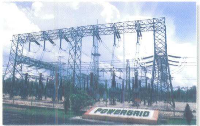
A view of 400 kV Durgapur sub-station switchyard
