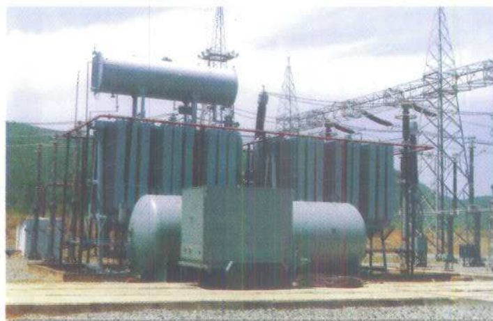
View of Auto-Transformer
