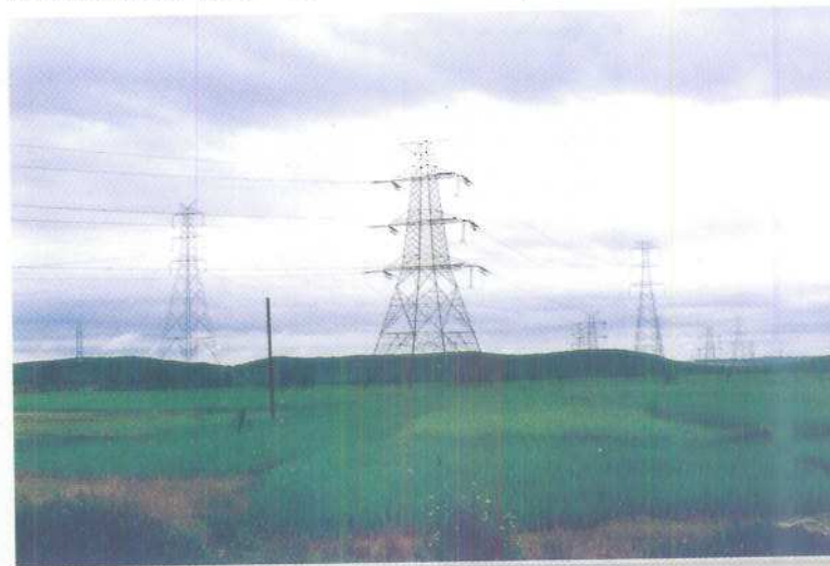
View of two 400 kV lines - Durgapur-Jamshedpur and Maithon-Jamshedpur lines
