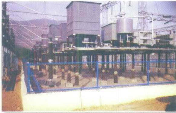
Series capacitors at Kishenpur S/S on 220 kV D/C Kishenpur-Pampore line.
