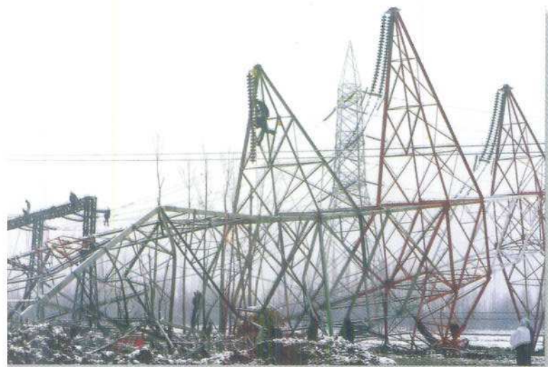
View of Blasted tower at Loc. No. 268 of 400 kV D/C Uri-Wagoora line on 15.1.2000.
