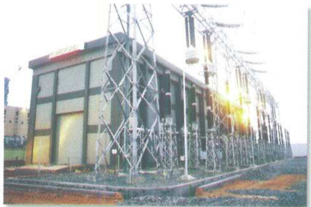
View of Kayamkulam Gas Insulated Sub-station
