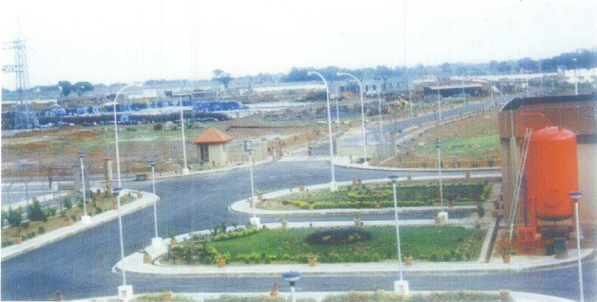
A view of 400/220 kV Raipur Sub-station
