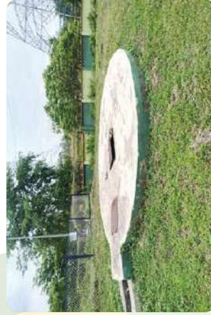
Pond at Bihar Sharif S/s for collection of Rainwater & Groundwater recharge
