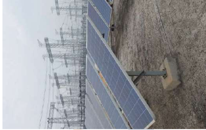
Solar PV at Bero S/s
