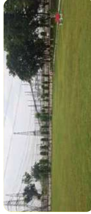
Green Landscaping at Biharsharif Substation
