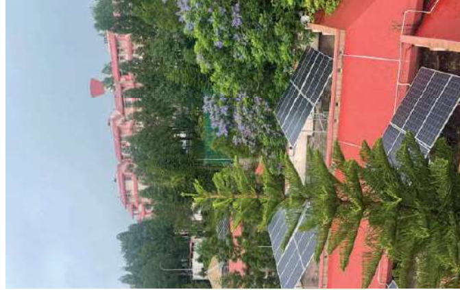
Solar PV at RHQ, Shillong
