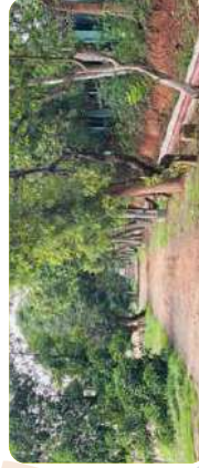
Green Cover at Jamshedpur Substation
